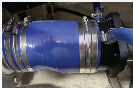
Closeup of the lip seal and misalignment.
