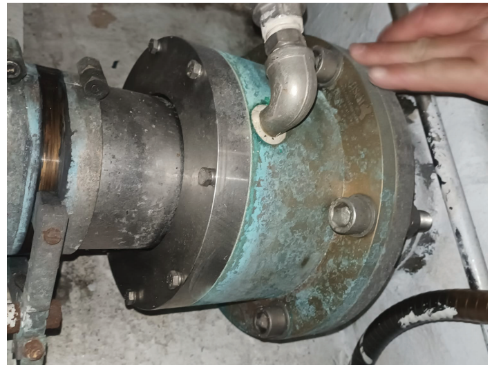
Original shaft seal in need of replacement.
